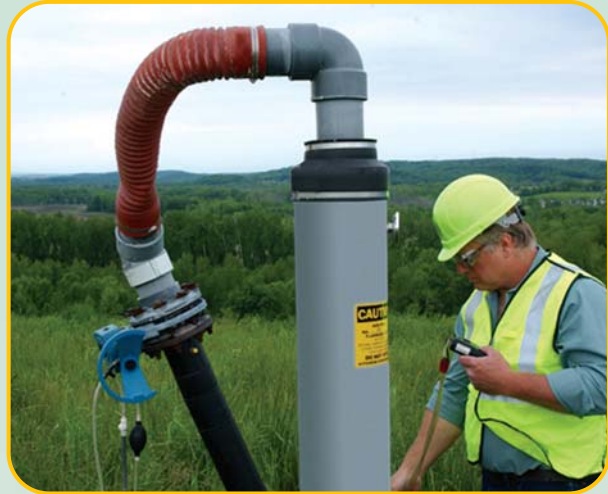
Advanced monitoring and control systems ensure that landfills remain at levels that meet even the strictest local, state or federal standards.
